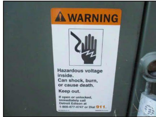
14. Tag affixed to pad transformer indicating ownership by Detroit Edison (DTE Energy).
