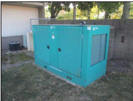
11. Emergency generator slightly west of the southwestern corner of the Property building.
