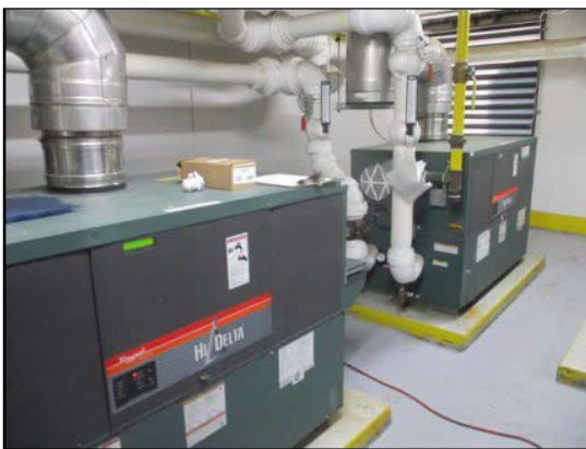
41. Typical boilers in the boiler room.
