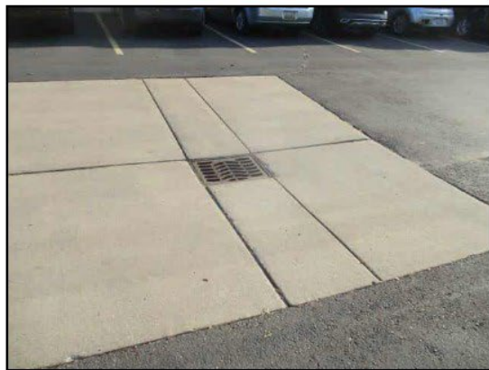
24. Typical storm water catch basin in the parking lot.
