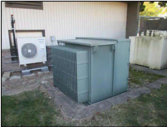
13. Pad-mounted transformer slightly west of the southwestern corner of the Property building.
