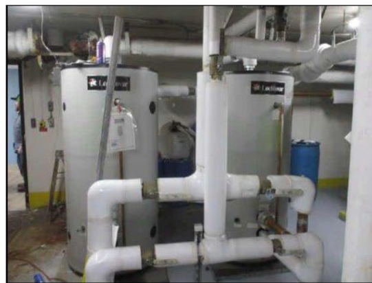
42. Hot water tanks in the boiler room.
