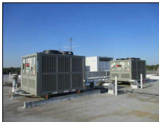
50. Newly installed chillers
