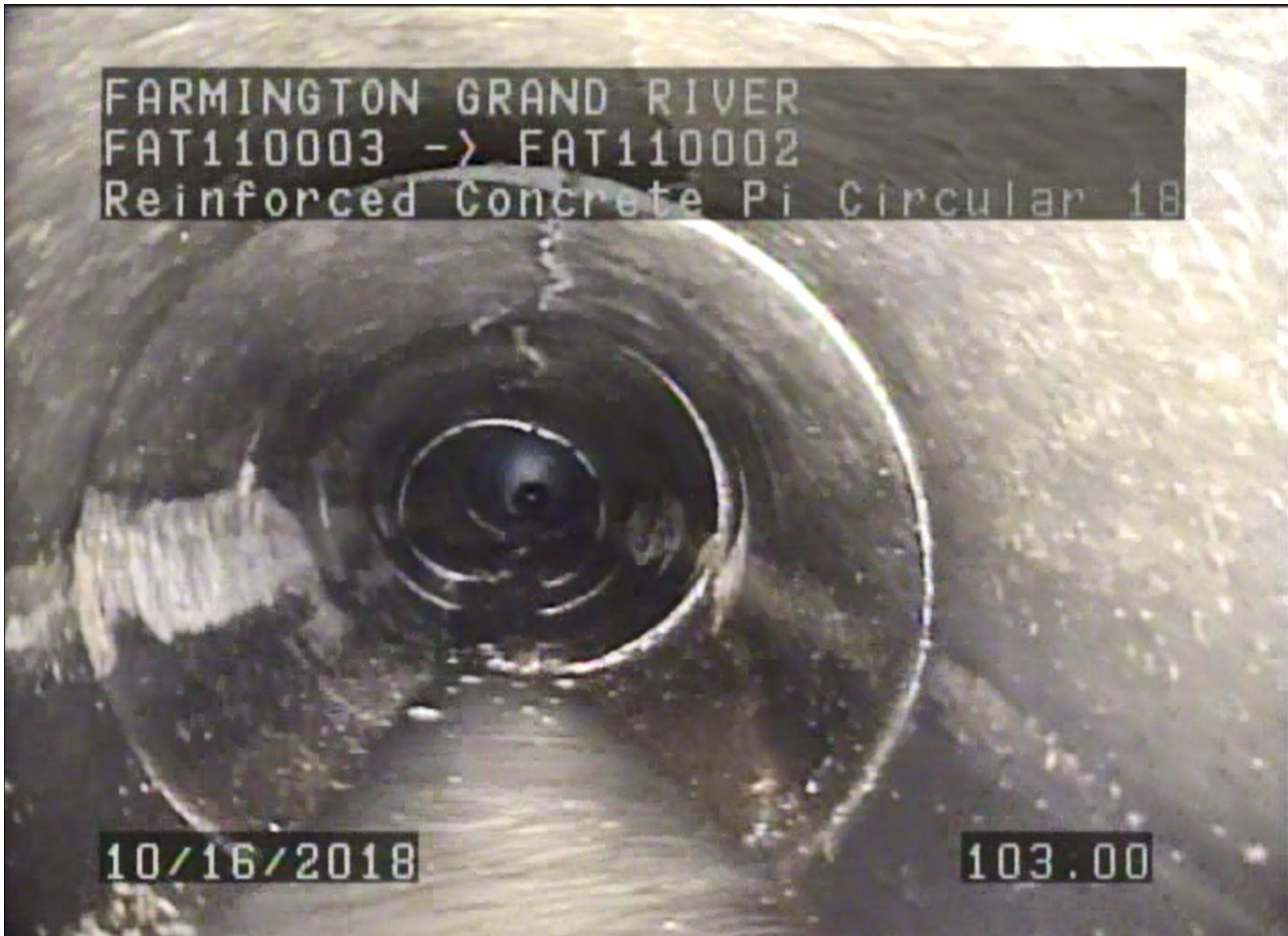
This internal photo of the pipe shows longitudinal fractures and cross-sectional deformation. CIPP lining recommended.
