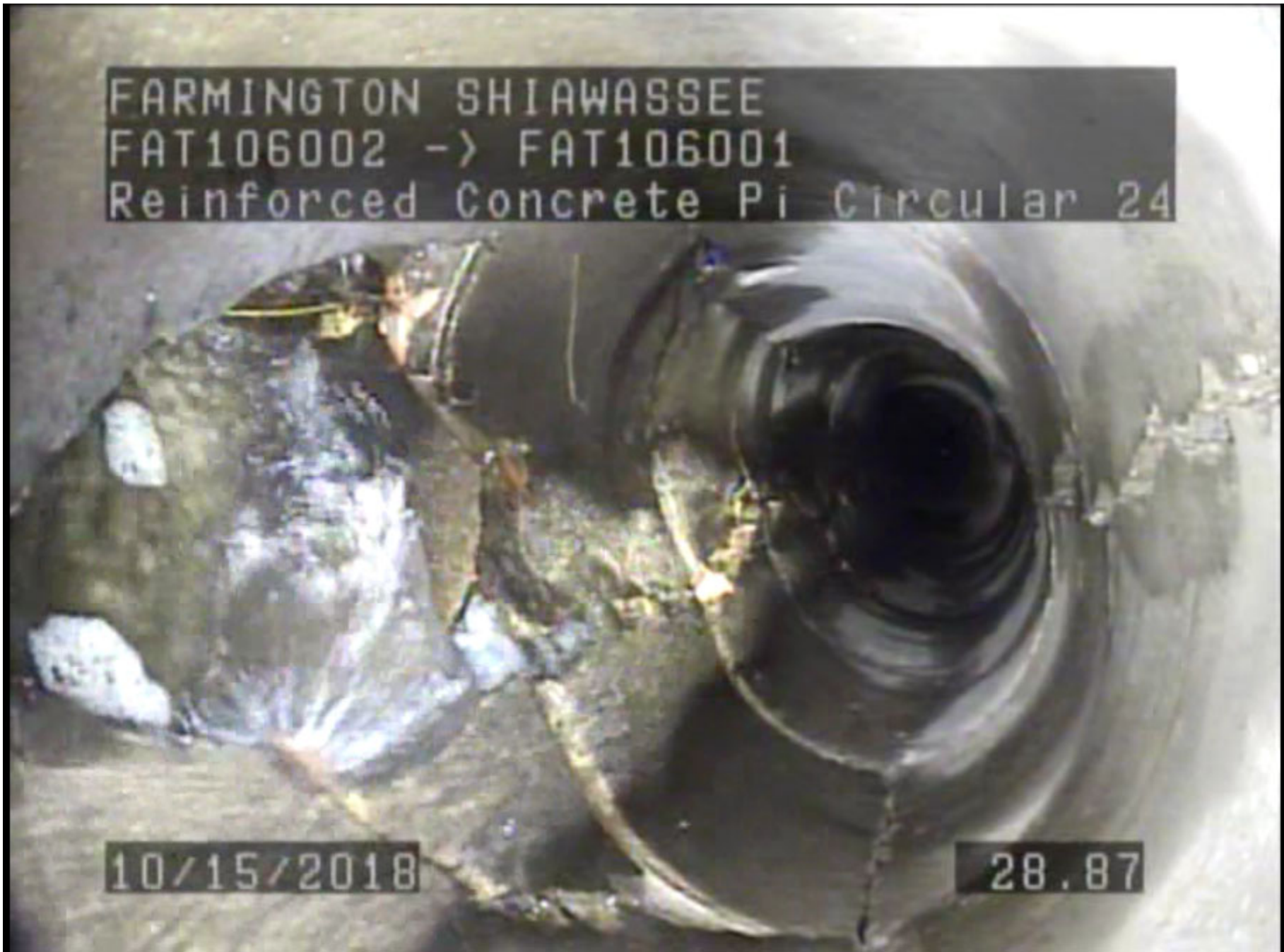
This internal photo of the pipe shows a Hole Void Visible that warrants a spot repair. Also visible is the cross-sectional deformation and longitudinal fractures, typical of this segment. CIPP lining of entire segment recommended.
