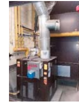
Furnace and HVAC Systems 20-40 Years Old
