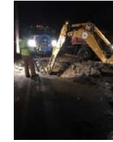
Water Main Break on Floral
