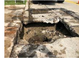
Catch Basin, Shiawassee
